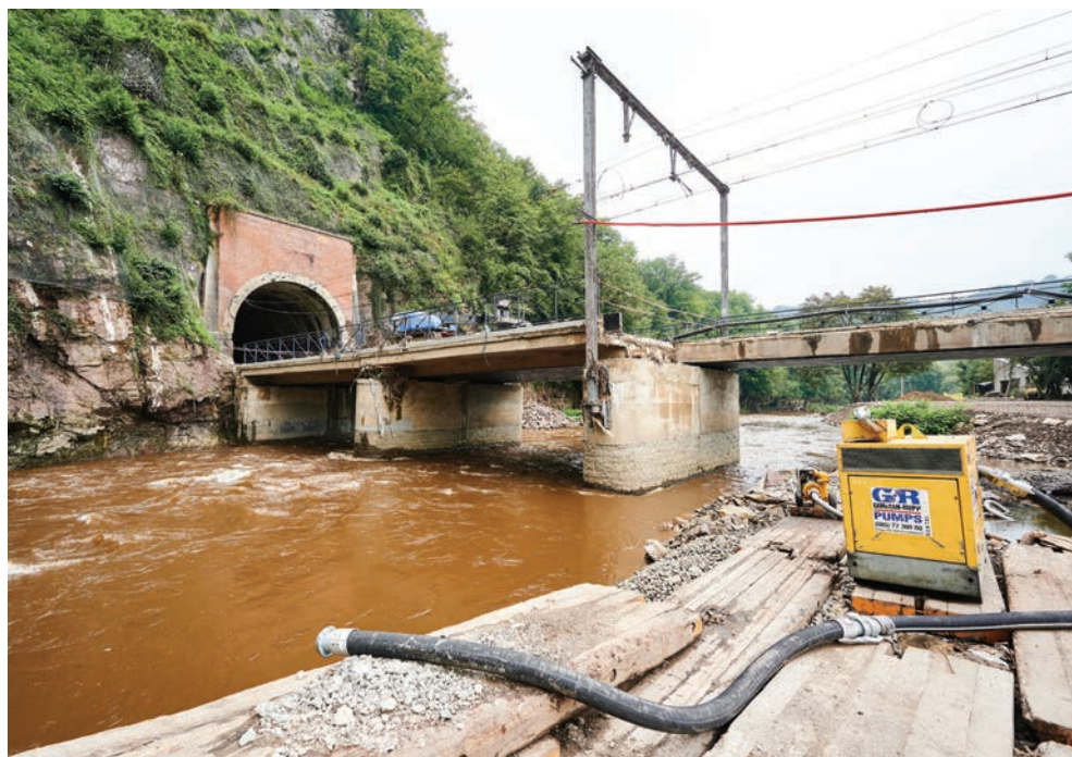
The Louheau bridge at Pepinster was damaged by same flood as the nearby Pepinster-Cité bridge on the Spa branch.
