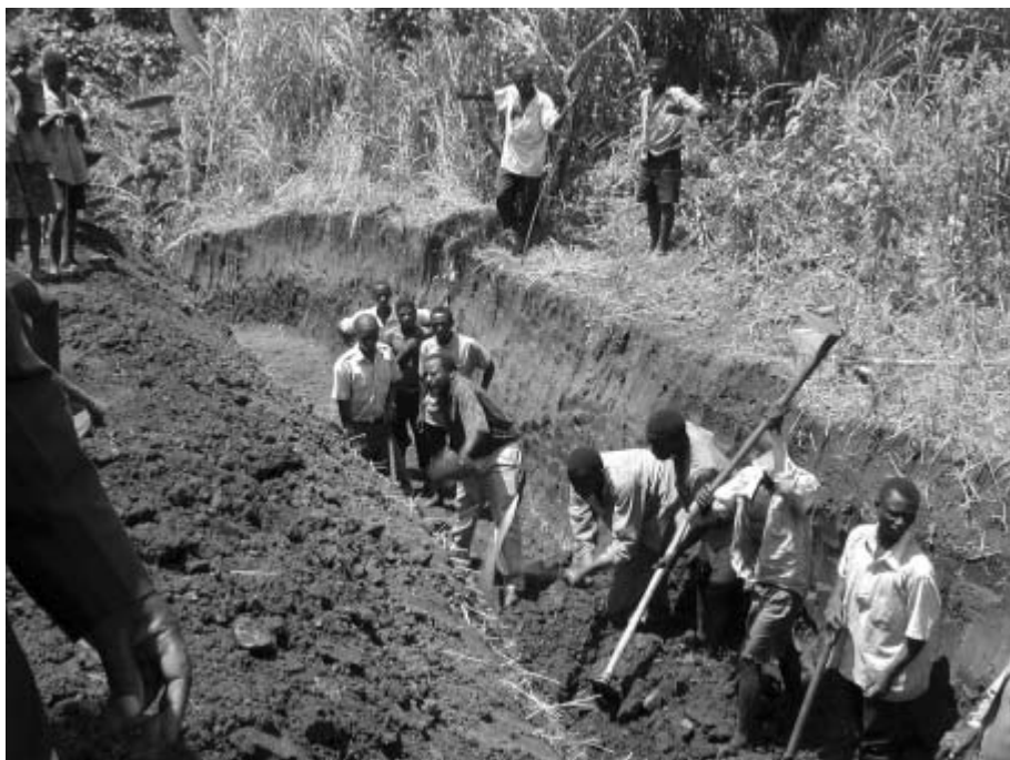
Figure 3: Digging a trench to prevent the elephants of Kibale National Park from encroaching into the surrounding cultivated fields. (Courtesy Purna Chetri)
