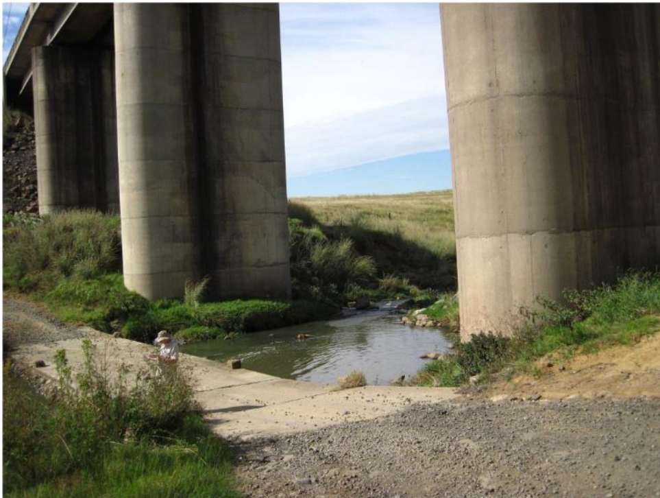
Figure 18: The south-westerly flowing Klein Drinkwater Spruit under the railway bridge on Portion 3.
