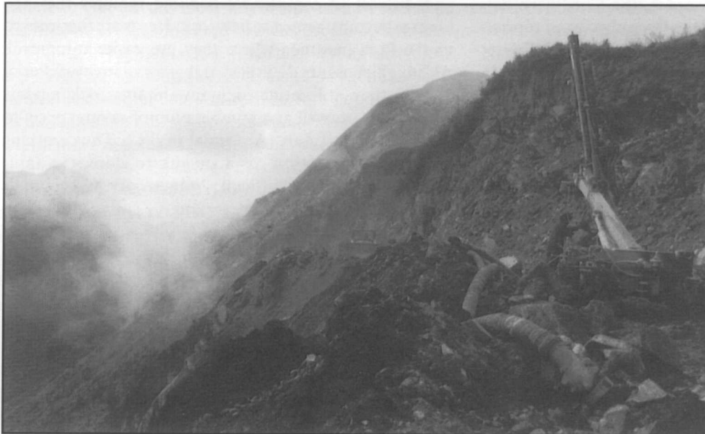
Figure 2.4b. Construction of highway through the Purshi sector of Sangay N.P., threatening 600km 2 of virgin Andean forest.
