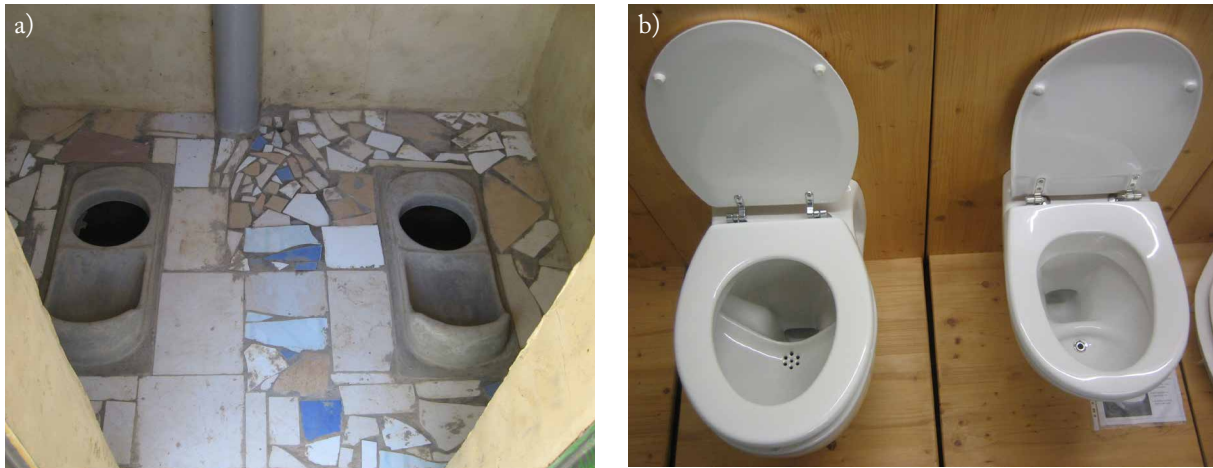
Figure 6.4 Urine, free from fecal contamination, can be used as a safe source of phosphorus fertiliser for crops. a) Urine diverting toilets in Nepal. Urine is collected in the basin at the front, whilst faeces collect in the hole at the back. b) Left: urine-diversion flush toilet by Roediger (Germany). A valve opens only when the user is seated to prevent flushing water from draining into the urine tank. Right: urine diversion flush toilet by Gustavsberg (Sweden). In this design no valve is used, this allows a little bit of flushing water to enter the urine pipe to avoid potential clogging of assemblies. Photographs courtesy of The Sustainable Sanitation Alliance (SuSanA).
