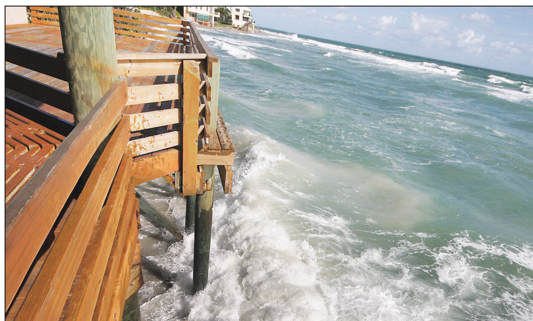
Waves crash against the pilings of the deck above Bathtub Reef Beach, where beachgoers used to lie in the sun. Erosion over the last few years has deemed the beach, unsafe and hit is currently closed to the public.
